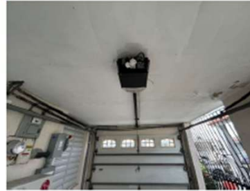
Carport - Gate motor
